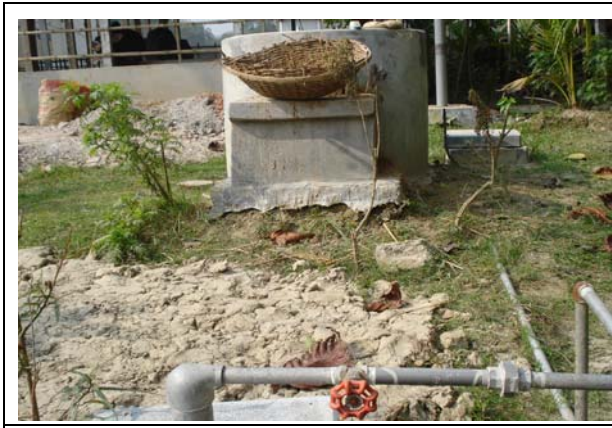
Underground Gas distribution line
