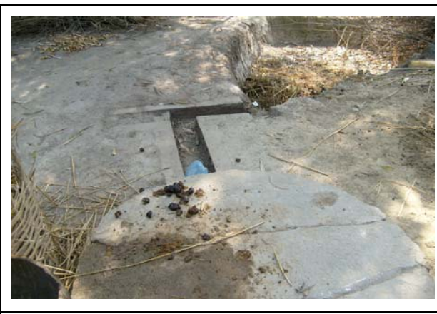
An inactive plant
