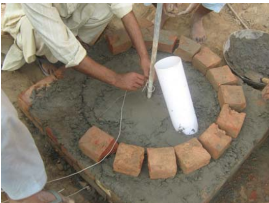
Photograph 4-11: Masonry work continuing to construct compartment to be used for feeding of animal manure into the biodigester unit
