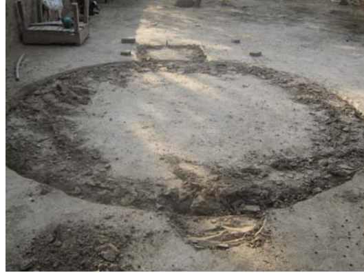
Photograph 4-2: Marking of dimensions for biogas unit prior to start of excavation work
