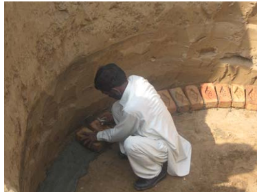
Photograph 4-4: Brick lining being conducted by the mason at the base of the biogas unit
