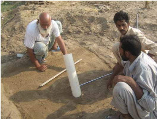
Photograph 4-9: Inlet pipe for feeding of the animal manure into the biodigester unit
