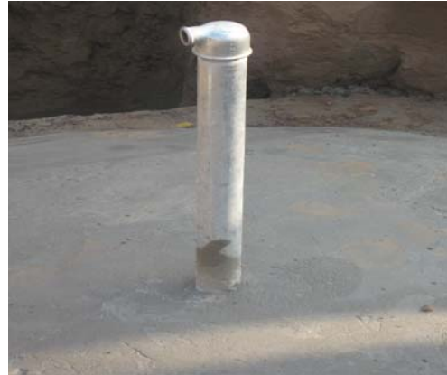
Photograph 4-14: Outlet pipe on top of biodigester to be used for piping of the gas produced to the household appliances
