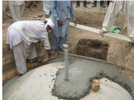
Photograph 4-10: Concrete being laid on the biodigester dome to ensure no leakage of gas takes place during operation
