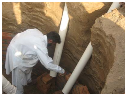
Photograph 4-6: Inlet pipes for feeding of the animal manure into the biogas unit being inserted
