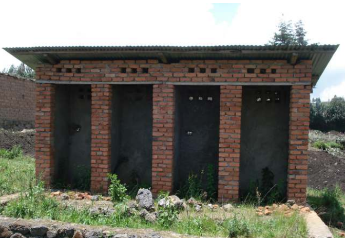
Who is accountable for dysfunctional latrines?
