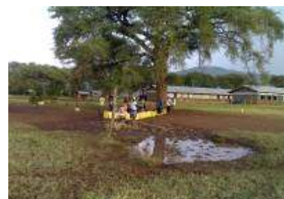
A poorly maintained borehole at Ngenge primary school
